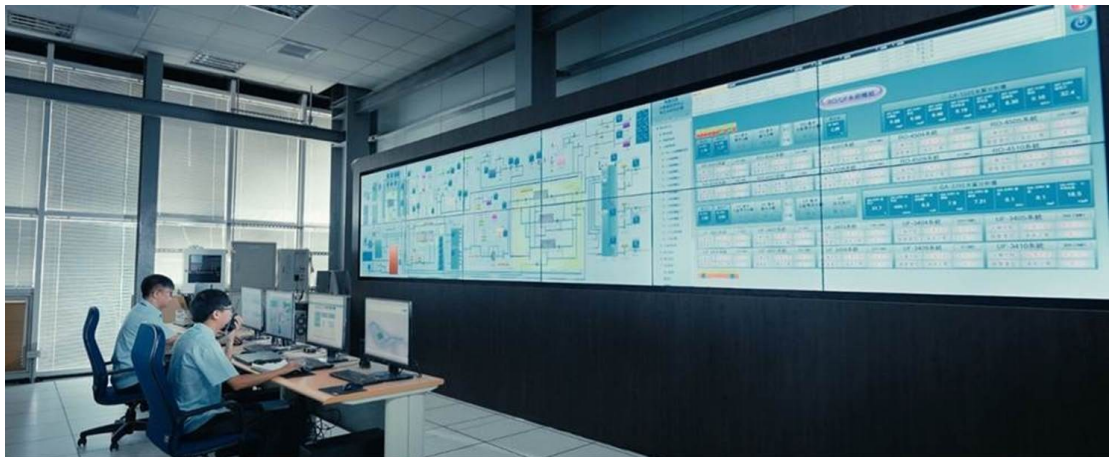
Bao Ding Reclaimed Water develops Taiwan's first AI-monitored smart reclaimed water plant
